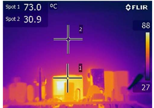
Figure 32 – 195 VAC, Full Load. Spot 1: Transformer Core. Spot 2: Ambient.
